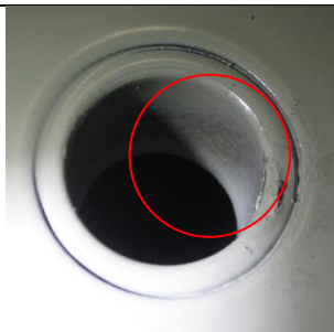
Figure 8 – Thin/missing paint in enclosure/case or panel mounting hole that exposes less than 1/2” of bare metal.
