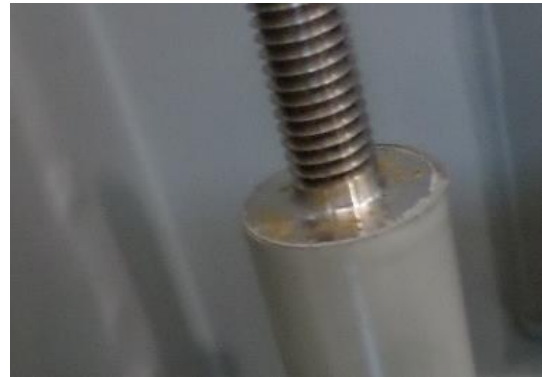
Figure 19 – Area of Rust Greater Than 1/8 in. Wide
