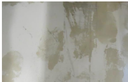
Figure 40 – Discolored Plating (Yellow)
