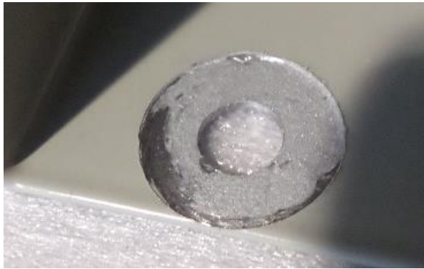
Figure 18 – Area Missing Zinc Paint Greater Than 1/8 in. Wide
