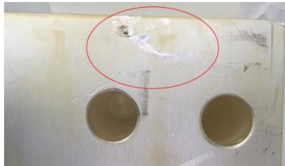
Figure 38 – Damage in Joint Area
